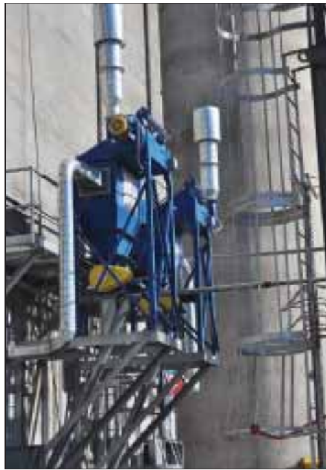
Donaldson Torit cyclones mounted near the receiving pits. Much of the project focused around beefing up dust collection systems.
